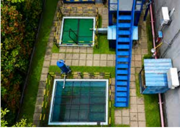
RPC Factory - Reuse of wastewater
