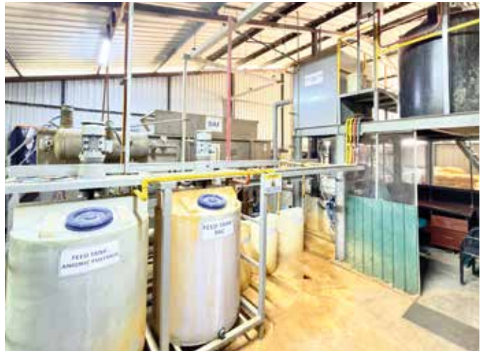
CIC Poultry - Water purification and reuse system
