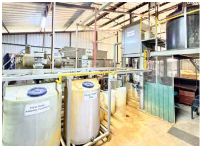
CIC Poultry - Water purification and reuse system
