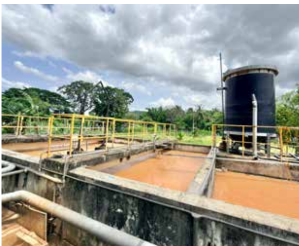
CIC Dairies Factory - Reuse of wastewater
